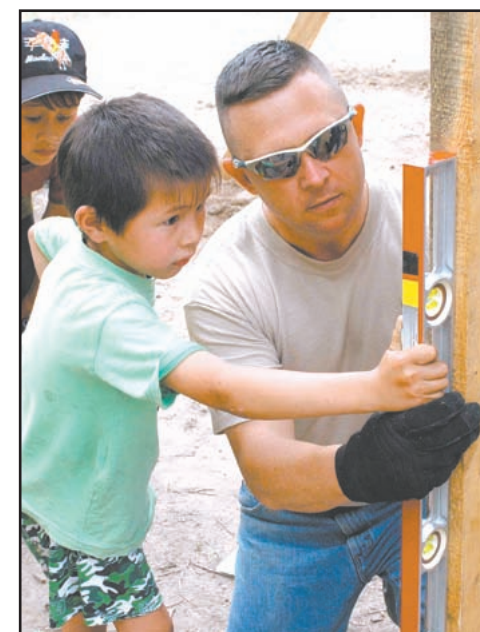
Tech Sgt. William Gordon, 376th Expeditionary Security Forces Squadron, shows an Oktobersky Village School student how to ensure a part of the playground is leveled. Members of the 376 SFS and 376th Civil Engineer Squadron visited the school to begin construction of a new children's playground. Sergeant Gordon is deployed from the 482nd Security Forces Squadron, Homestead ARB, Fla.
